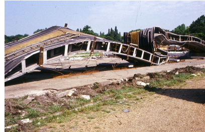
Figure 6: The collapsed arch
