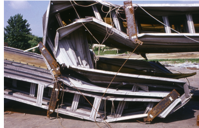
Figure 7: The collapsed arch detail
